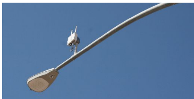
DSRC radio installed on a traffic signal luminaire arm.
